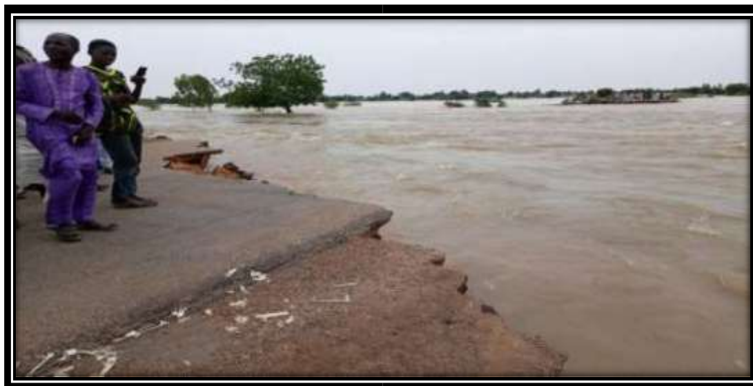
Plate I Picture of the Collapsed Hadejia Gujungu Road
