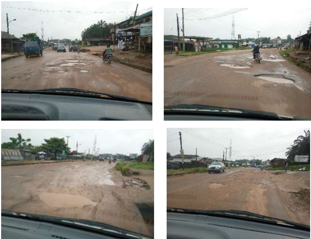
Figure 2. Photo of some of the pothole spots captured
