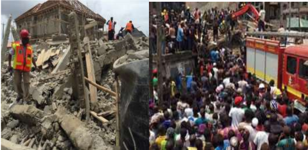
Plate 1 Showing: A Cross Section of a Collapse Building in Lekki Area of Lagos
