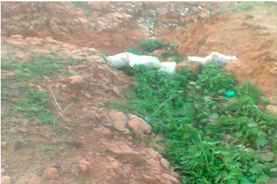
Plate 3: Use of sand in sacks as means of controlling soil erosion in the area Source: Fieldwork, 2014
